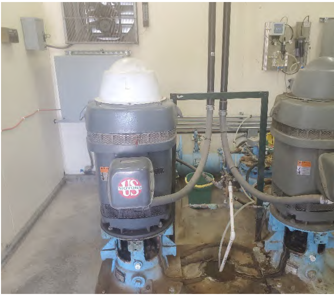
Photo 1. Booster Pump Station
