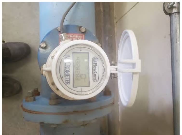
Photo 4. Master Flow Meter for Booster Pump Station
